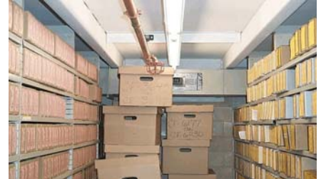
Figure 1: Stacked materials too high blocking sprinkler's range.
