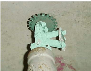
Figure 4. Corroded sprinkler in an area where chlorine chemicals were stored.
