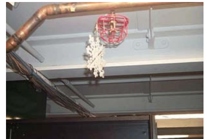
Figure 3. Decoration hanging on sprinkler guard.
