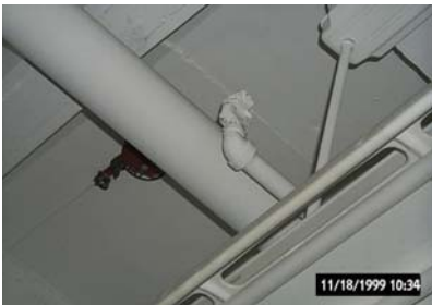
Figure 2 Completely covered sprinkler
